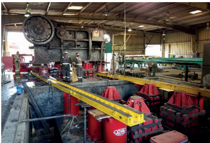
The pipe bending machine is raised 6 ft. out of a pit before being skidded over 60 ft.
