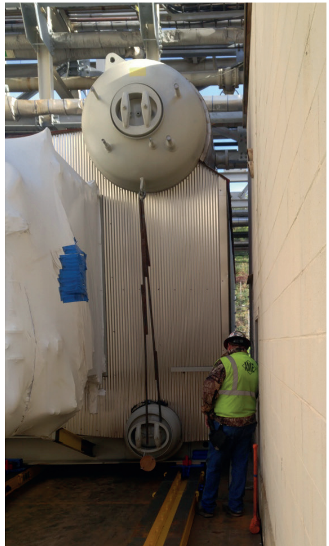
AME personnel keep a close eye on the path of the boiler during the slide.
